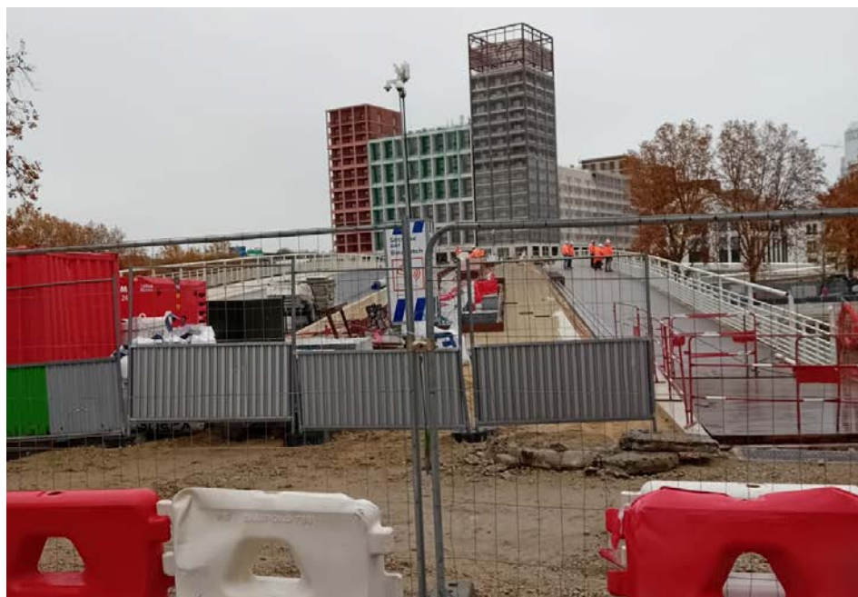
Construction of the Passerelle Seine planned to be completed before the games
