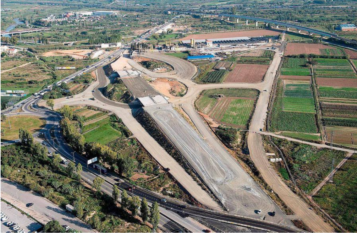
The B-25 expressway project is planned to take over the historical C-245 road between Sant Boi and Cornellà in the Lower Llobregat Agricultural Park increasing the physical disconnection between both cities © Generalitat de Catalunya
