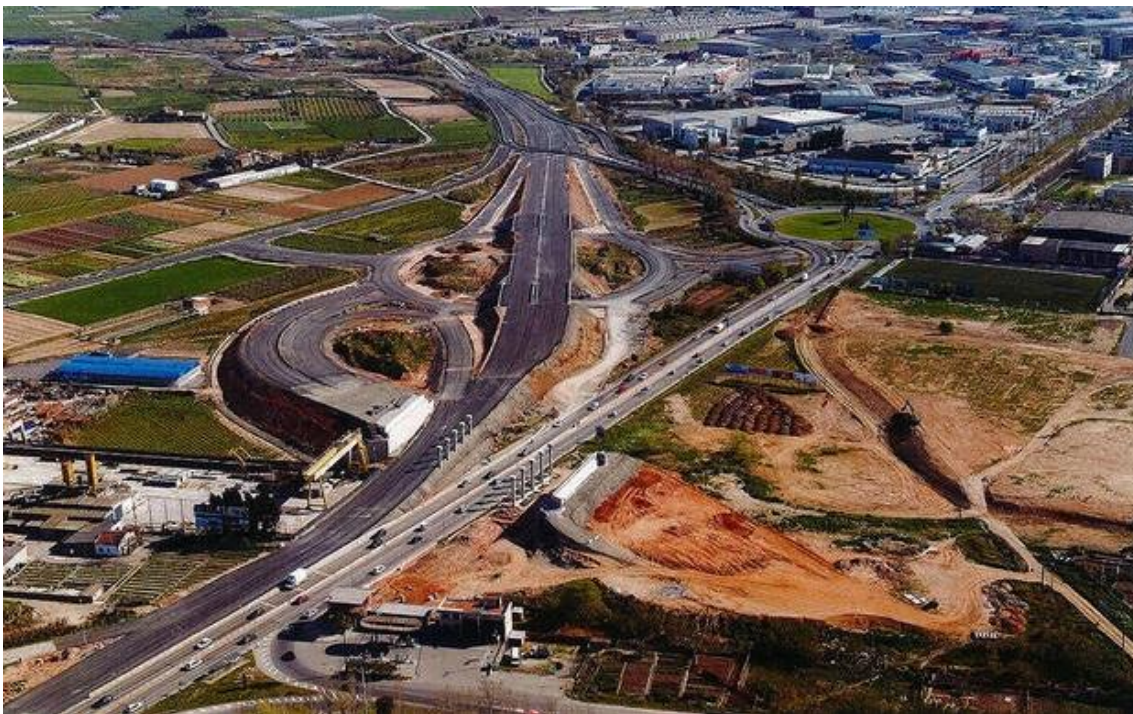
The 4 lane (2+2) C-245 in the Llobregat plain (looking south) between Cornellà and Sant Boi, with the future B-25 expressway bypass in construction and the commercial developments south of the road © Generalitat de Catalunya
